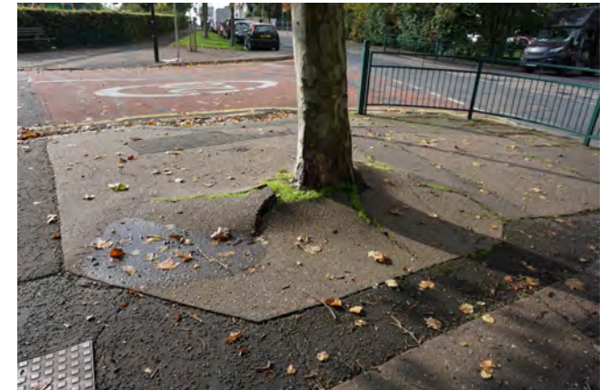
Damaged pavement surfaces through tree root growth
