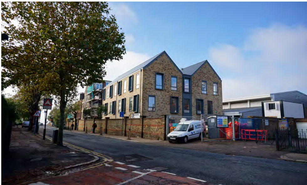
New warehouse style extension to St. Bernard's High School being built opposite Avenue Baptist Church
