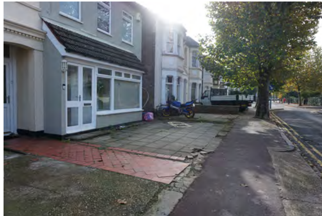
Damaged surfaces to private driveways
