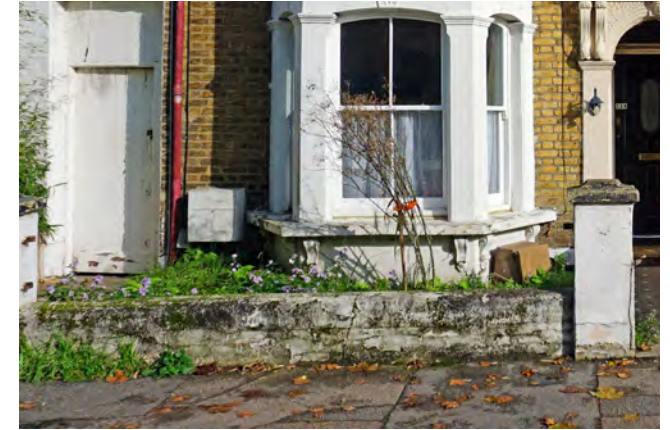
Boundary wall in poor decorative condition
