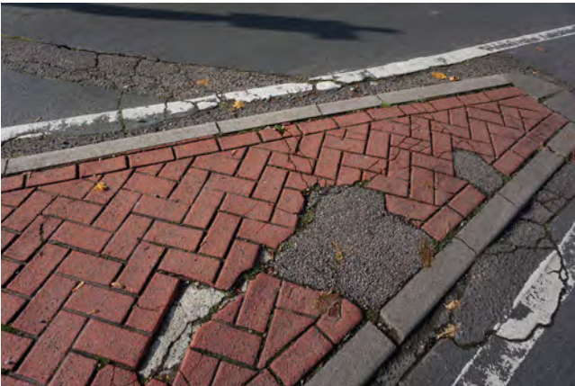
Brick effect paving, which is damaged and patched in tarmac
