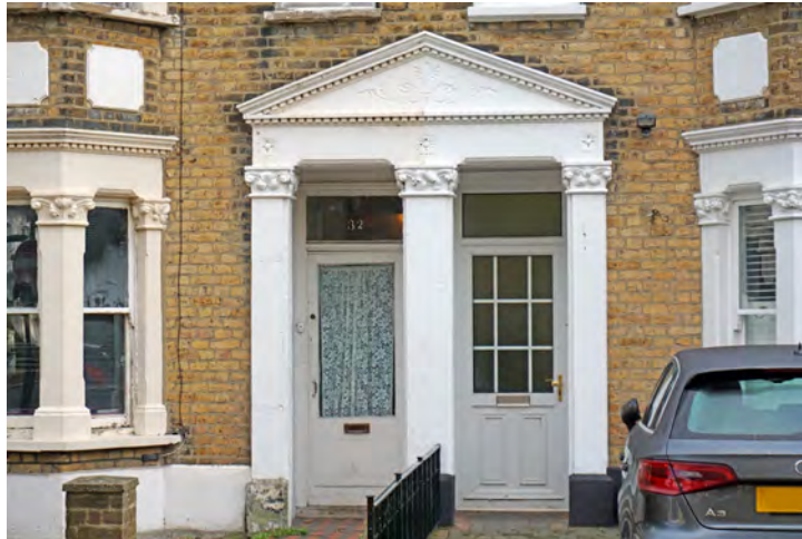
Replacement front doors which do not have the same character as the original timber ones with stained glass
