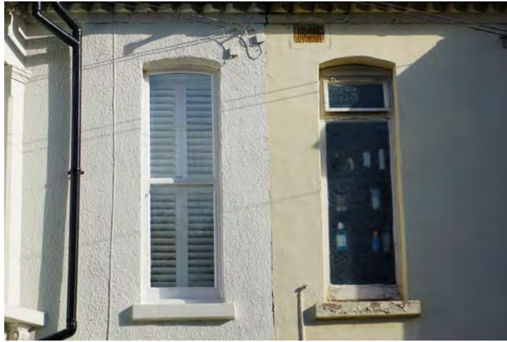
Inappropriate casement window on the right, compared with a traditional sash on the left
