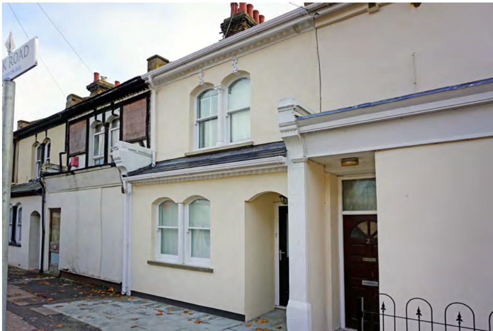
Park Road shopping parade, now residential with some units in need of repair and renovation.
