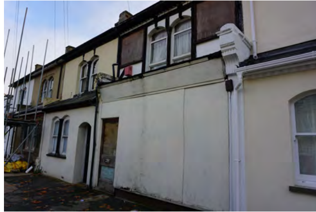
Poor decorative condition of buildings on Park Road
