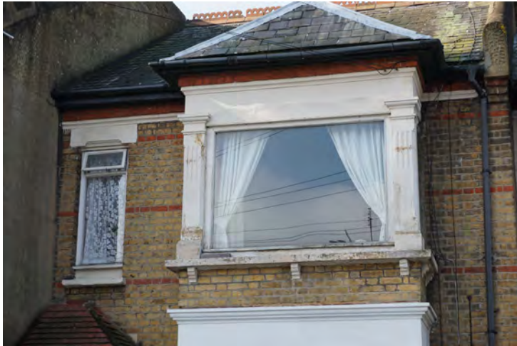
Inappropriate picture window and casement window replacing sash windows
